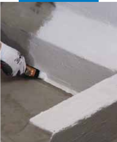
Triblock P applied to blend in the joint between a floor slab and a vertical wall
