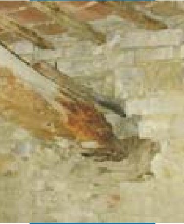
Damaged beams at the support
