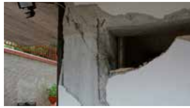
Failure of beam-pillar joints
