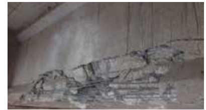
Beams hit by impact loads
