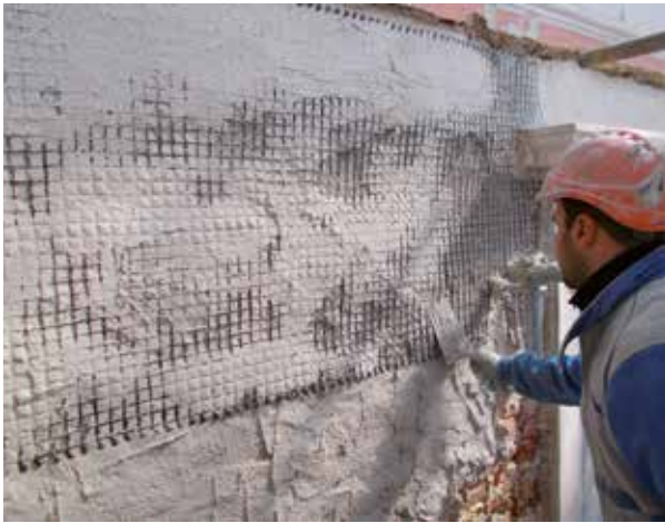
Application of a compact strengthening system to increase the shear-tensile strength of bay walls
