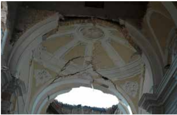
Collapse of masonry vaults
