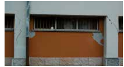
Failure of stocky pillars
