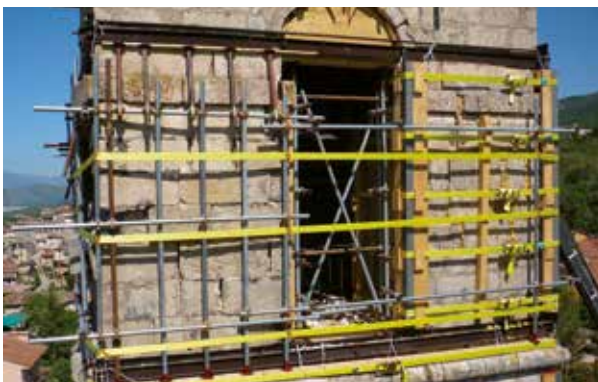
Damage to bell towers
