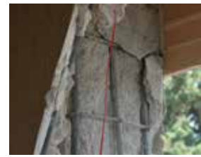
Instability of steel reinforcement
