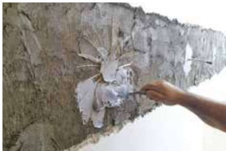
Application of an FRCM system to prevent collapse of dividing and buffer walls
