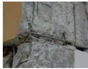
Defects in second concrete casting
