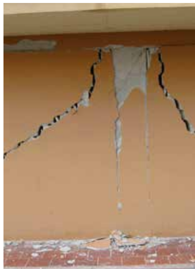
Shear failure of partition walls
