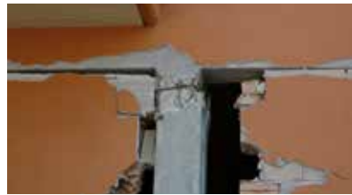
Shear failure of pillars
