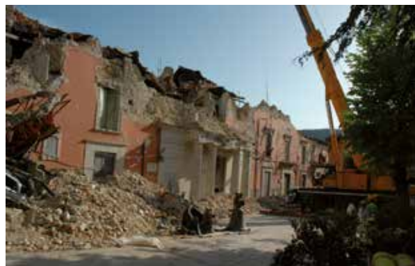
Masonry with poor mechanical properties
