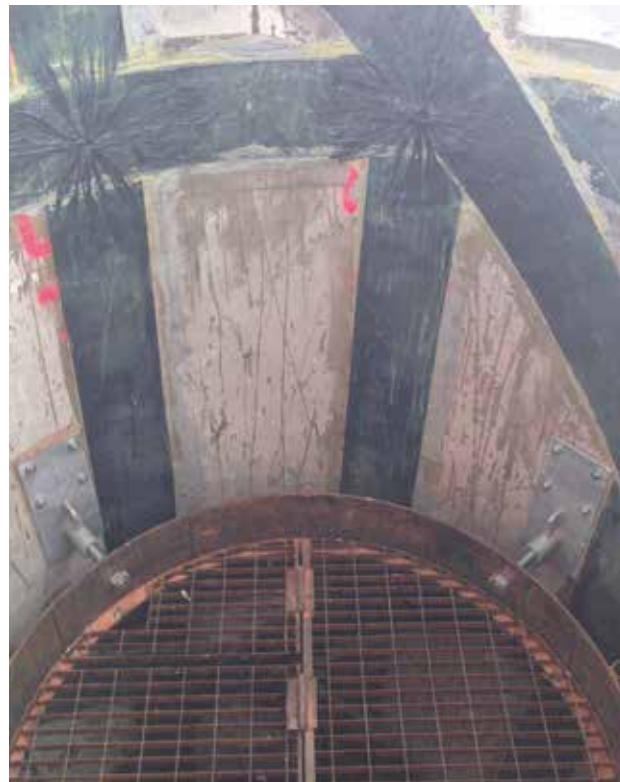
Strengthening of a brickwork chimney with MAPEWRAP C SYSTEM – Villaggio Crespi d'Adda
