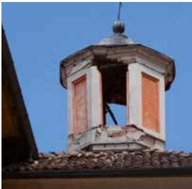
Damage to skylights
