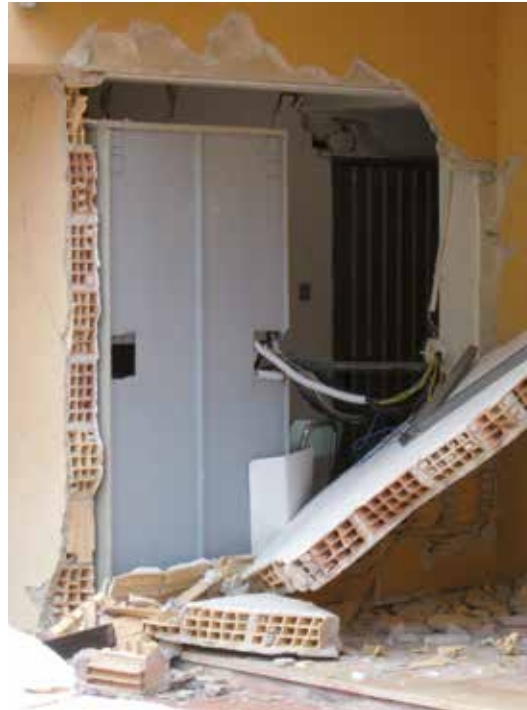
Overturning of internal partition walls
