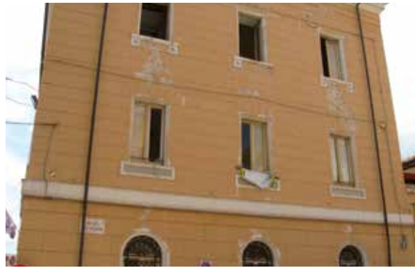
Shear cracks in load-bearing walls
