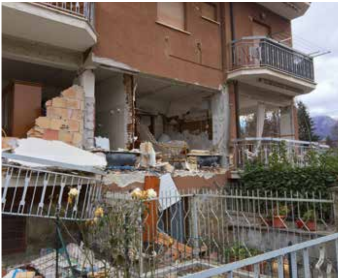
Collapse of external buffer walls
